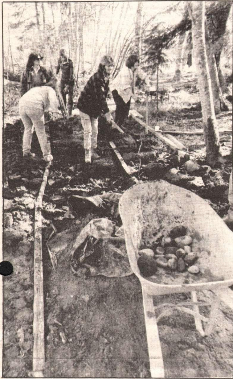
Job-Trac crews are currently working on creation of linear park for Ganges Creek, and on new washroom facilities at Centennial Park. Above, employees landscape portion of linear park.
