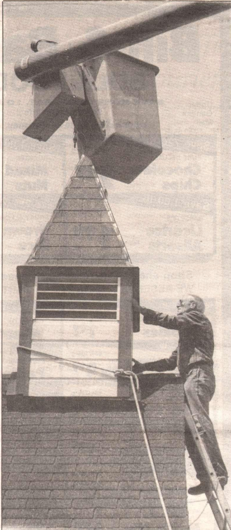
Replica of original Burgoyne United Church bell tower was added to building last week as a project to mark structure's centennial. Above left, Peninsula Tree Service employee Don Gallagher keeps a line on 'tower'
