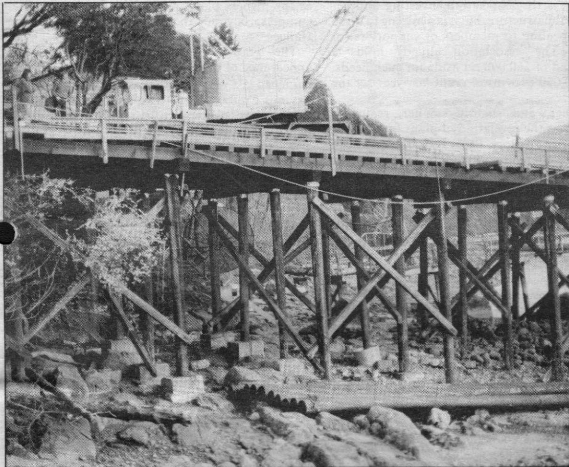
Vesuvius ferry dock is currently being upgraded. Timbers that are replaced will not go to Cy Peck
