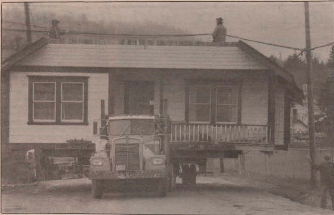
Workmen hoist lines across Rainbow Road to ensure house they helped move will clear the
