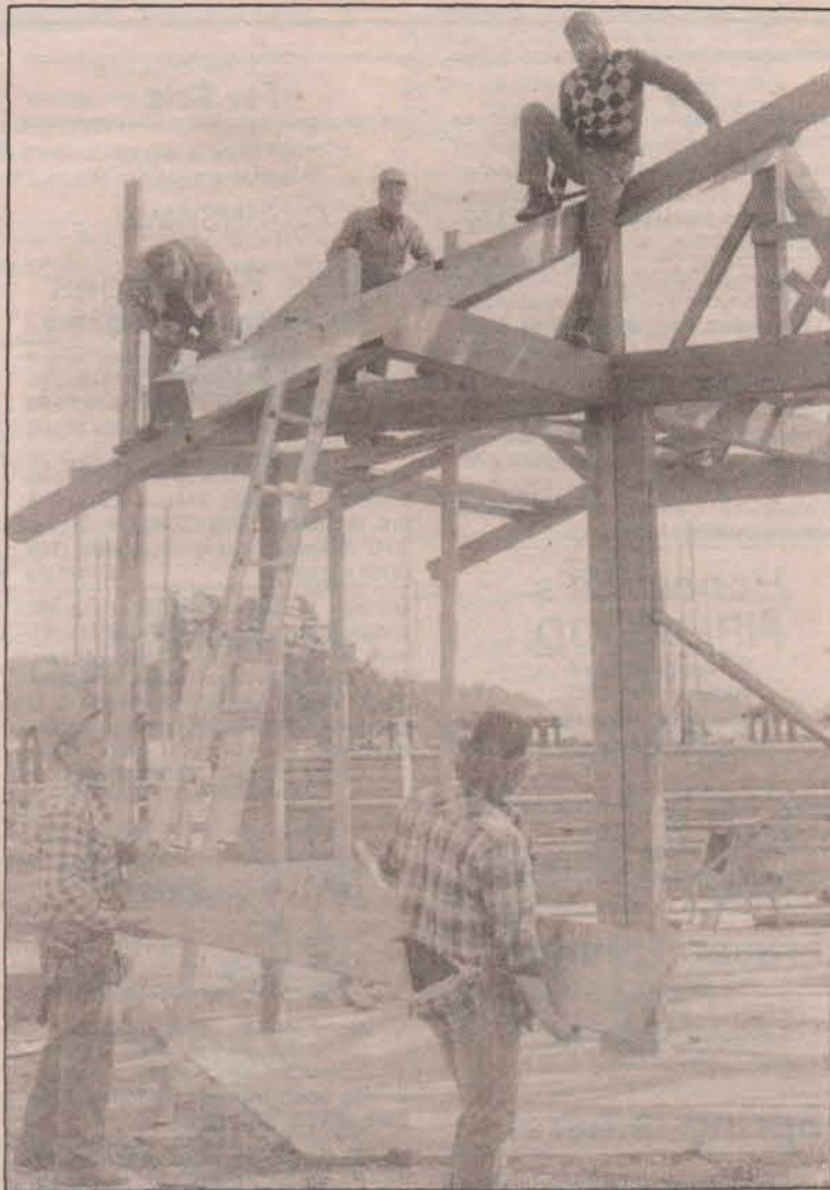
Work has resumed on the Centennial Park bandshell project in downtown Ganges, which organizers hope to have ready in time for this summer's Sea Capers celebration. Volunteer help is
