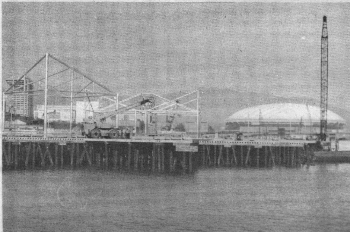
A general view of the Expo site shows the buildings already started and piles under the area
