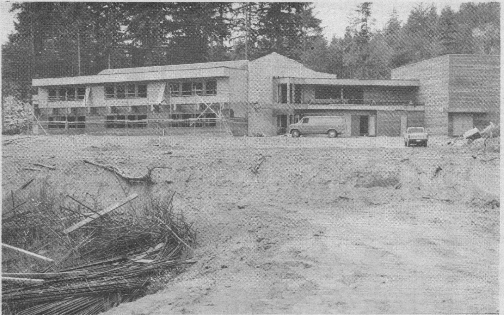
Fulford Elementary School nears completion. The six classrooms can be seen on the left of the structure while a portion of the gymnasium is
