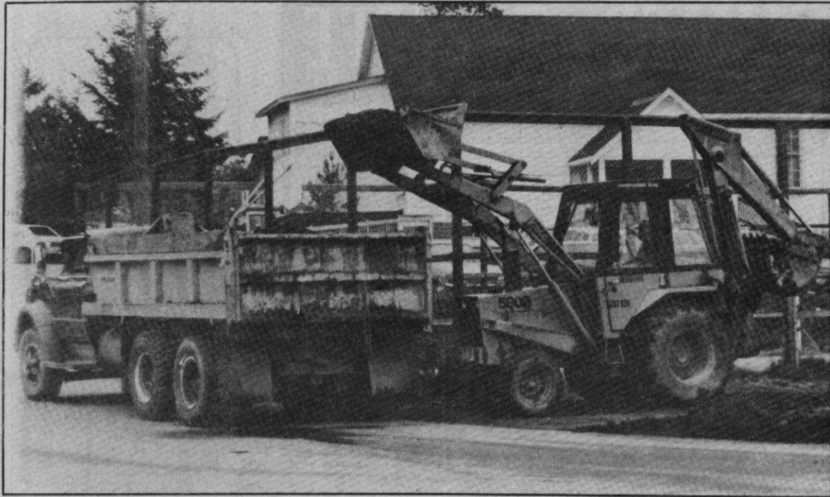
Gravel is delivered for the parking lot in the play area near the Gulf Islands School Board office. The 21 interim plan to bring greater safety parking spaces are the first step in an to the Ganges school complex.
