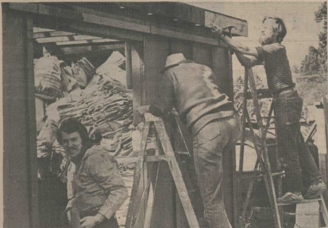
The finishing touches are applied to the Recycling Shed. Busy at work on the structure are Franz Beyk, left, Beth Hill with her back to the camera and Nick Gilbert.
