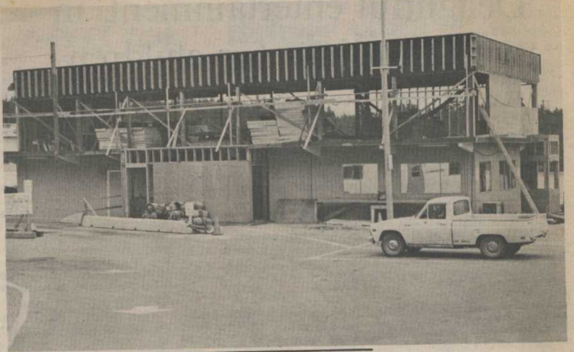
Addition to the ferry terminal building at Long Harbour is beginning to take shape. Second storey being added to the building will provide more office space for the ferry corporation.
