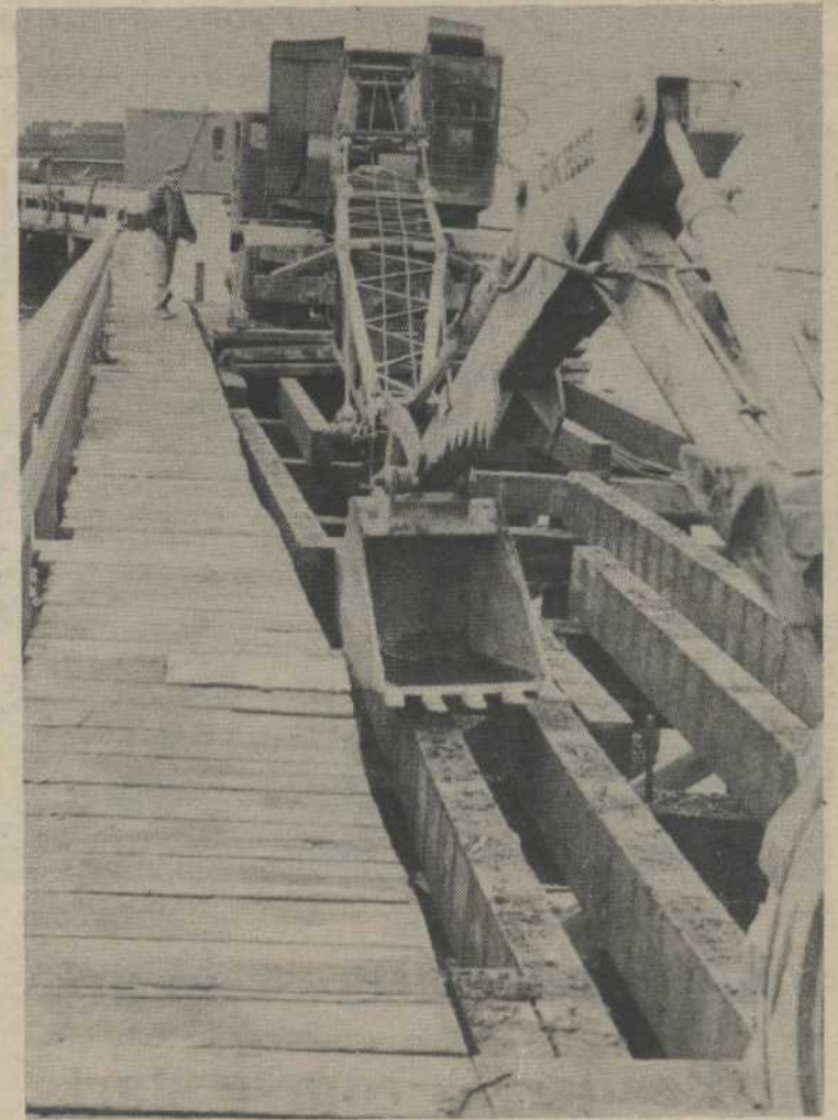
Rebuilding of the Miner's Bay wharf at Mayne Island commenced last week; Dolphin Pile Driving, of Sidney, is doing the $87,000 job. Some Mayne Islanders have been questioning the need for it.
