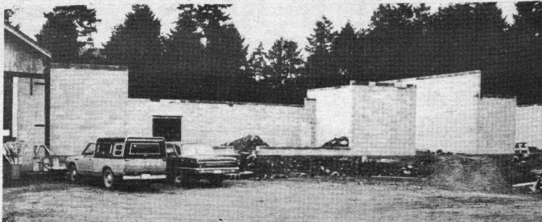
Walls are coming up fast at the new food market for Valcourt Business Centre at Ganges. Building on left is Foxglove Farms.
