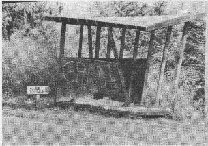
A few months ago, trustees of Gulf Islands School District were asked to erect a bus shed on Salt Spring but they were reluctant to do so because the sheds have a limited life-span. This shed on Vesuvius Bay Road has seen better days and has been placed on the market by some enterprising islander.
