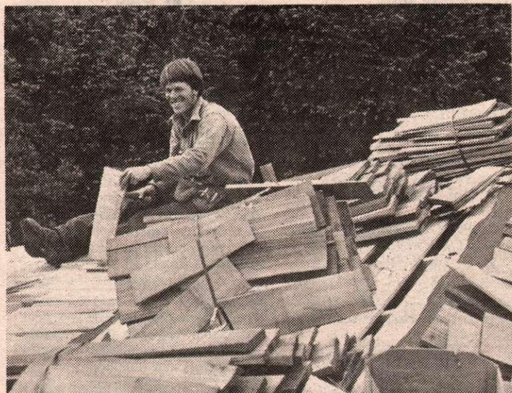
This week it is. same roof as brother Jack and Gordon Speed is roofing the helper Ernie.
