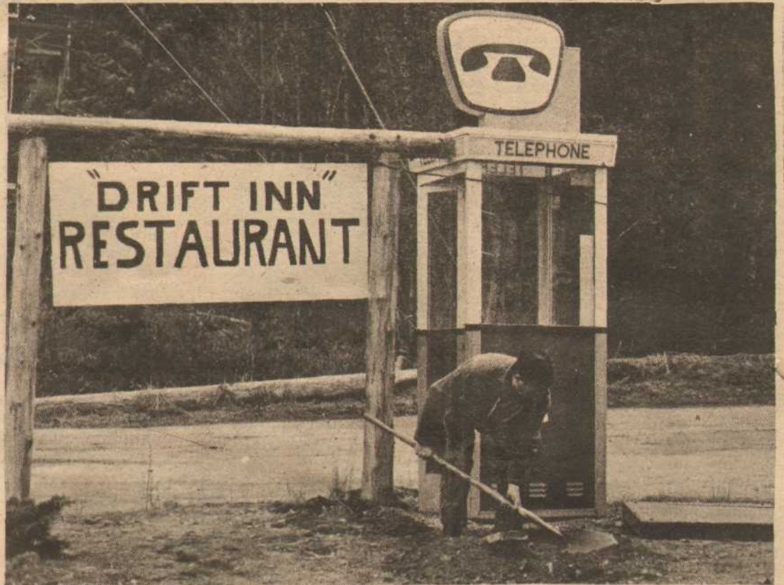
Installing new coin telephone for public convenience at Five Corners, on North Pender Island, is B. C. Tel Inst-
