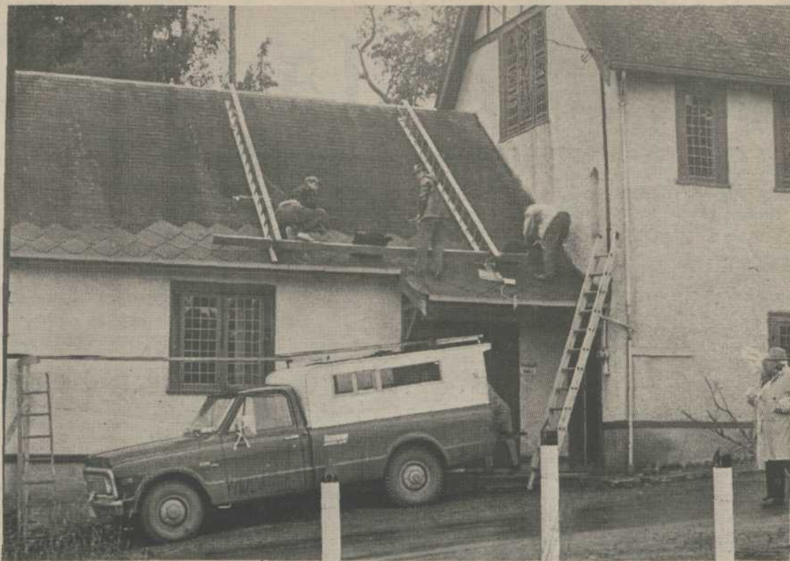
Even if it rains, the congregation of St. George's in Ganges will keep dry after roof repairs.
