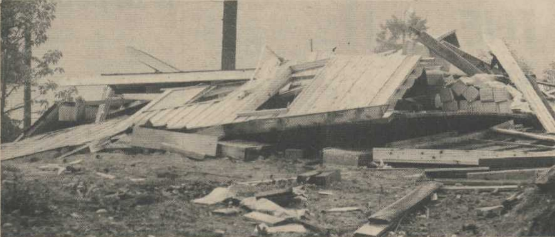
This house was almost ready for occupation on Sunday morning. It is located on St. Mary Highlands above St. Mary Lake.
