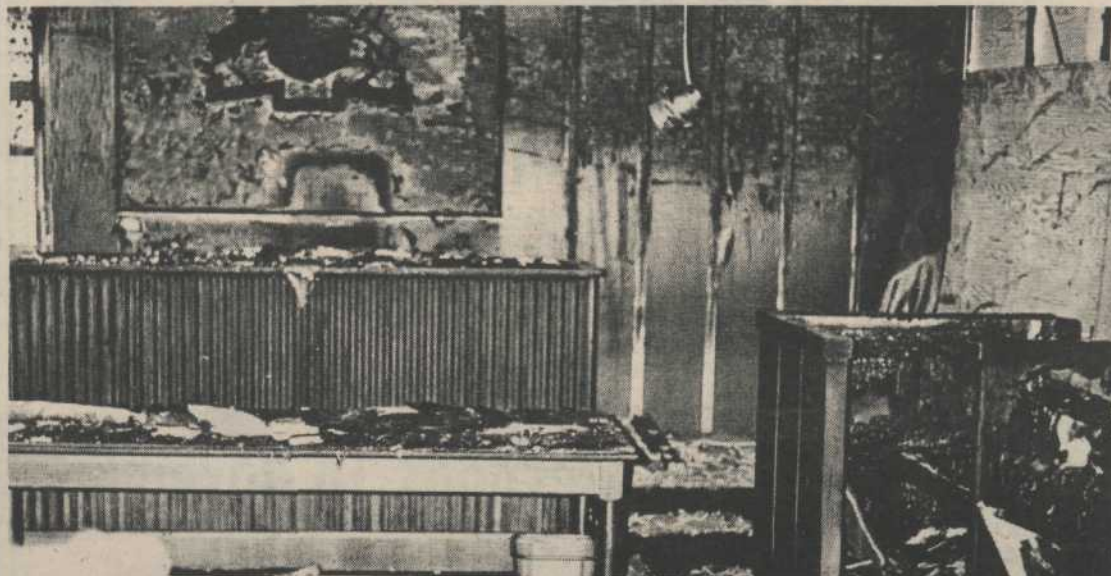
Interior of the Court Room after Saturday morning's fire had destroyed panelling and fittings.
