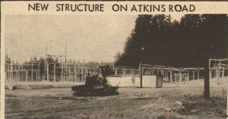
Something has been added on Atkins Road. New BC Hydro substation is shown in its near-finished state.
