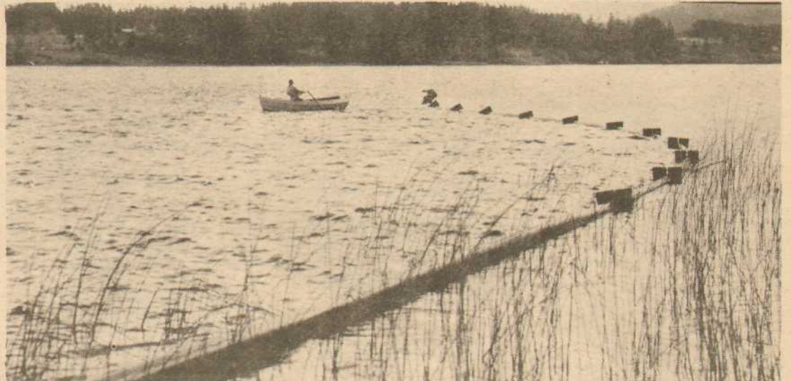
Lying on the water is the pipeline drawing water from St. Mary Lake. The attachments along the pipe are the weights which will hold it on the lake bottom. Peter Cartwright is at the oars.
