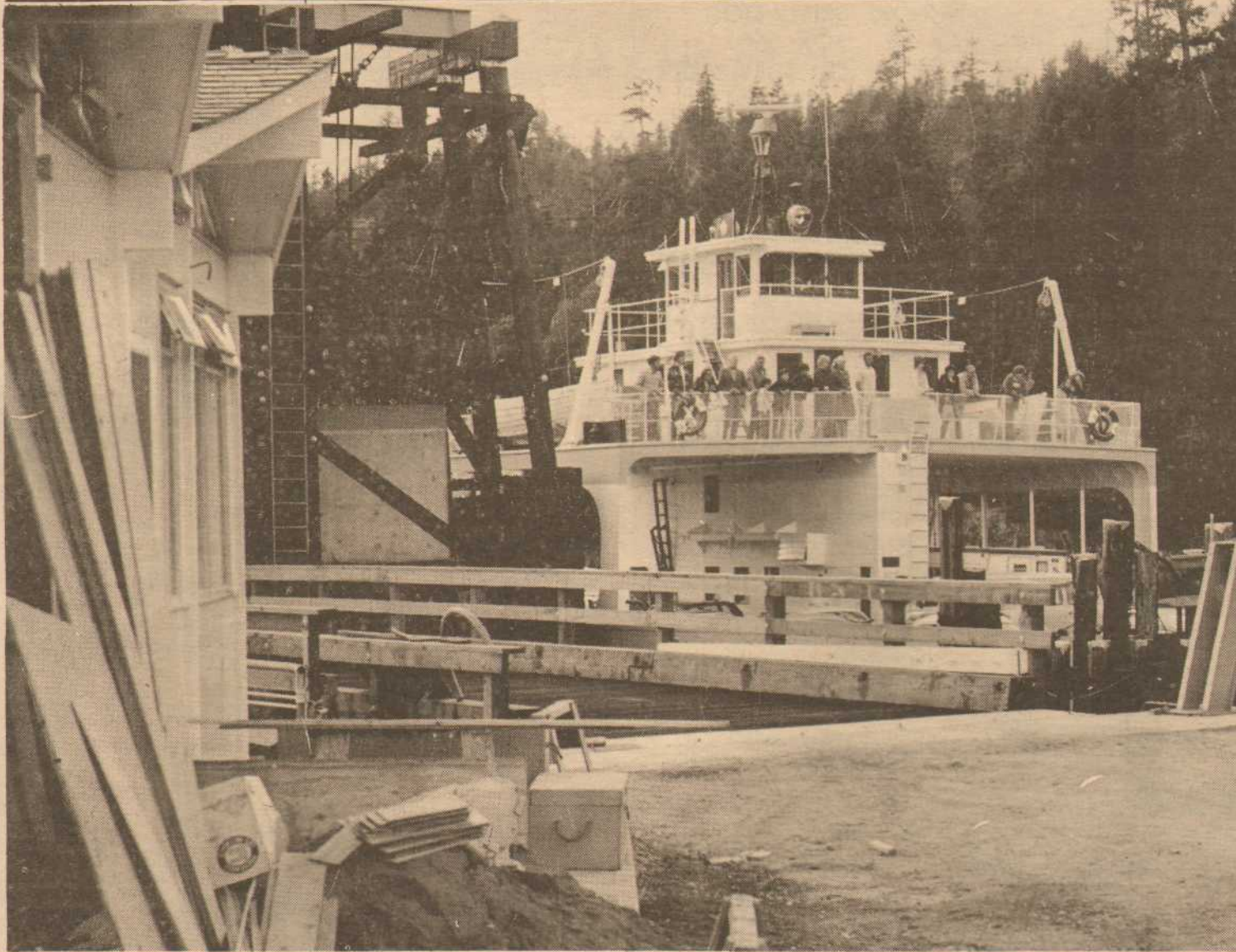
Salt Spring Queen is seen in this picture alongside the new wharf at Fulford. The vessel is filled and there were 26 cars lined up for the next trip when this picture was taken on Sunday evening. The new wharf structure may be seen as well as the new traffic signals.
