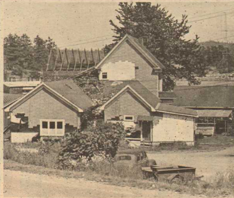
The large building, latterly used as Dr. Francis' Nursing Home, is shown as wrecking crews start their big job.
