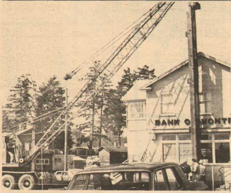
What a way to treat a bank! The pile driver has been and gone, driving the long posts into the ground as a basis for the new Bank of Montreal building in Ganges.
